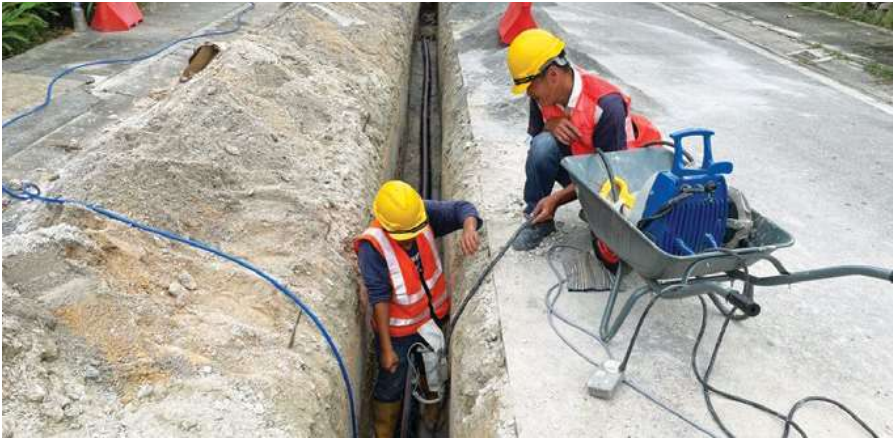
Laying of Vacuum Sewer & Telemetry Cable with total length of 4090m for rehabilitation works of vacuum sewerage system at Bandar Ambang Botanic
