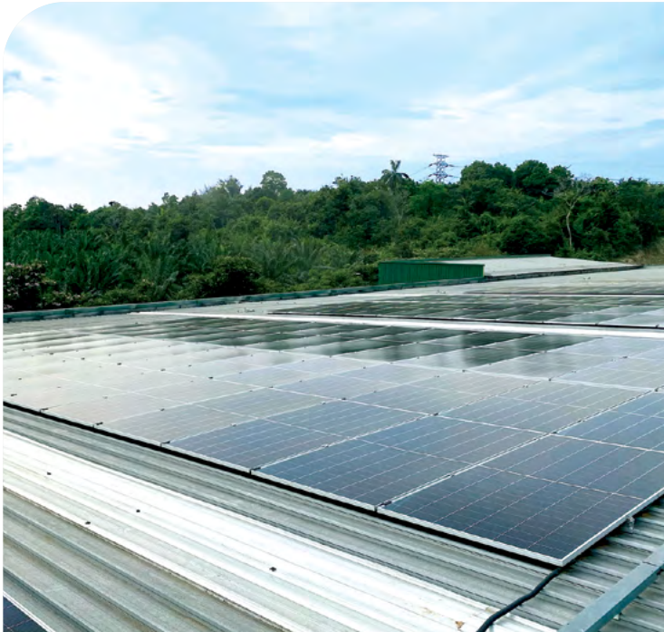
Rooftop solar panels on Heveaboard's building
