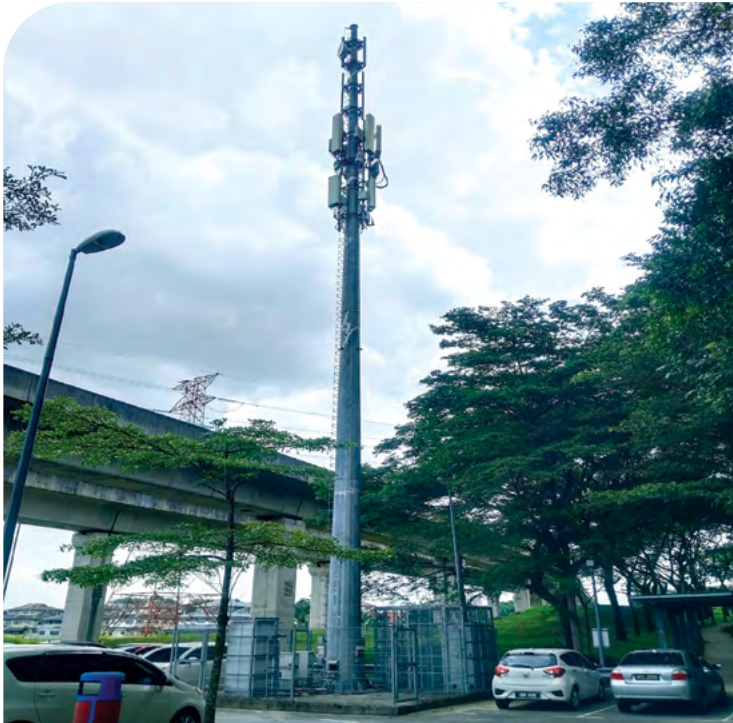
5G pole installed at LRT Lembah Subang
